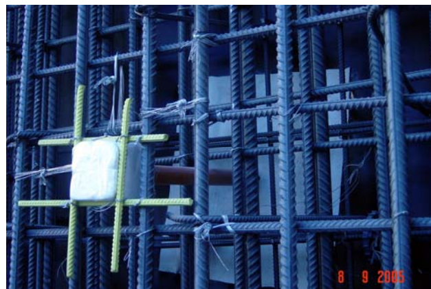
Protected inlet of Injection Pipe
